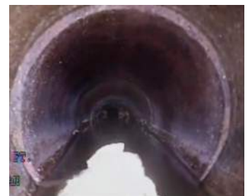
A hump in the the Main Street sewer near Brackenbury Square reduces capacity of the pipe.
