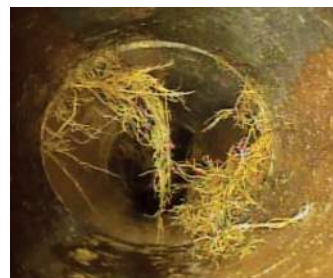
The local sewer in Main Street is susceptible to root intrusion creating on-going capacity and maintenance issues.
