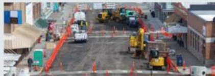
Main Street will be closed to vehicular traffic for the majority or all of the construction duration.
